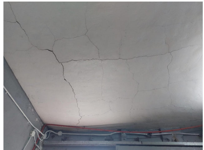
Figure 3: Cracks Formed under the Slab of Trench B.
